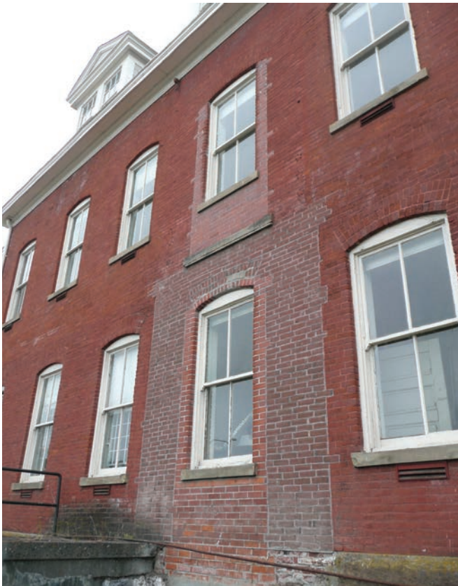
Windows at the Main Building's west elevation. Visible are the sections of infilled wall from an early connection to the Annex.
