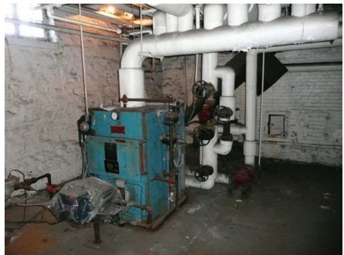
Existing boiler in the basement.
