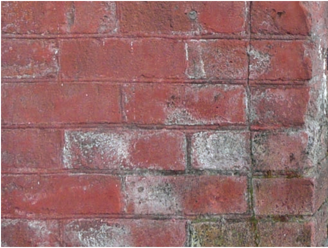
Close up of brick at the Main Building, showing the compromised weatherface due likely to sandblasting.
