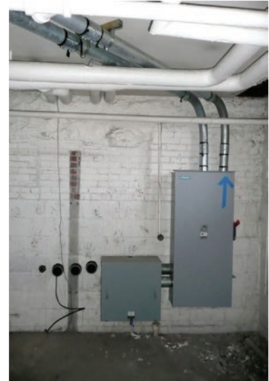
Electrical panels in the Annex.
