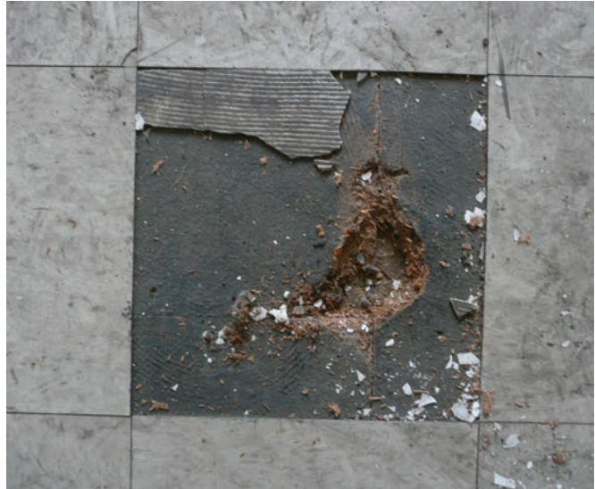
Layers of flooring, some of which are anticipated to contain hazardous materials.
