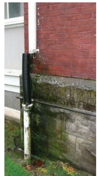
Damage to brick and stone due to disconnected downspout.
